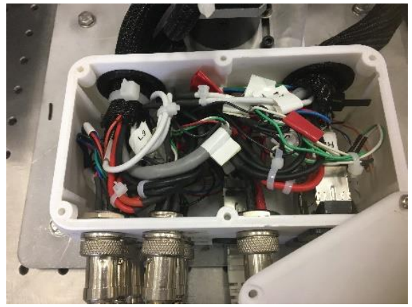
Fig 3. AR3 robot control box wiring
