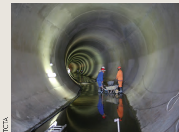
The conduit used for flood releases
