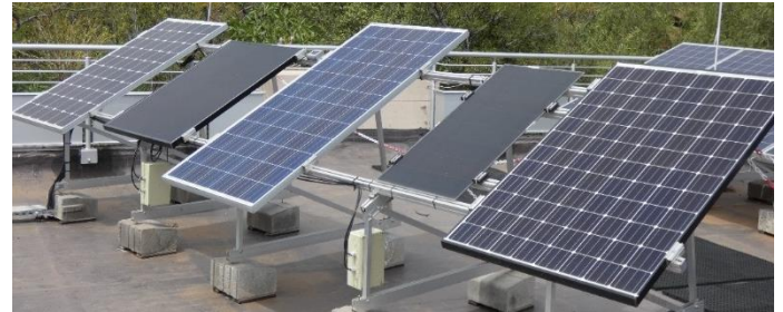
Fig. 4. Different PV module technologies under test at the CSIR Pretoria campus
