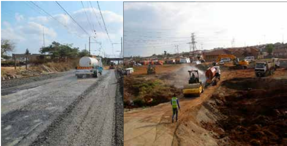
Figure 2: (Left and middle): Use of potable water in compaction (picture taken by G Mvelase at Transnet track formation layers construction), (Right): Video of use of water tanker sprayer on base layer to ensure optimum moisture content near King Shaka International Airport
