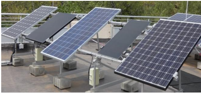
Fig. 1. Modules under test at the outdoor test facility on Building 34 in the CSIR Pretoria campus
