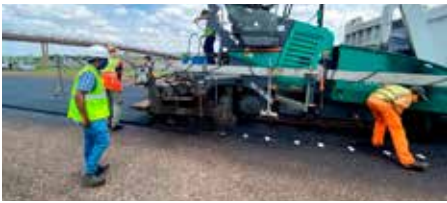
Figure 7: Construction of the HVS sections on road P159/1 (R80) in Gauteng, South Africa.
