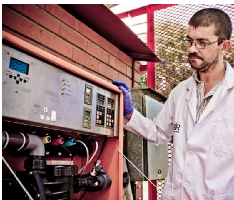
The CSIR's Calie Adlem inspecting a remote monitoring system installed at a water treatment plant.
