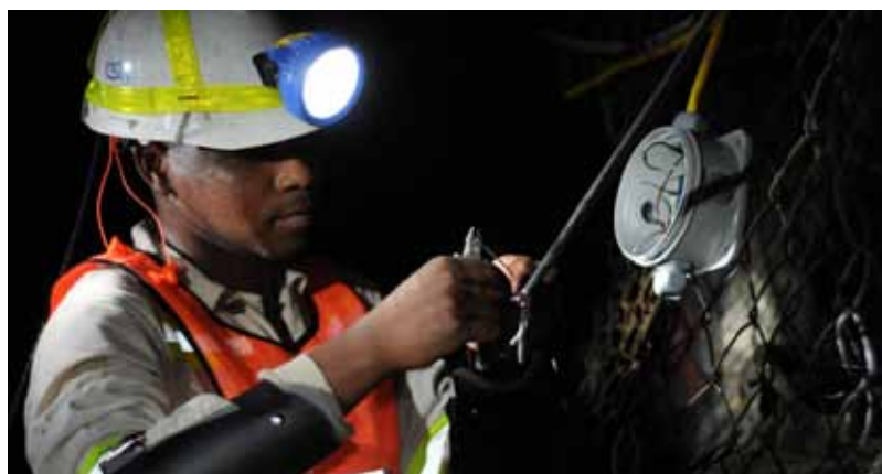
CSIR electrical engineer, Josias Nonyana, installs a connector to wires from a data logger, which connects to a geophone – an instrument used to measure seismic velocity. All collected data from the geophones are aggregated on the data logger. The data logger sends data to a server at the surface.
