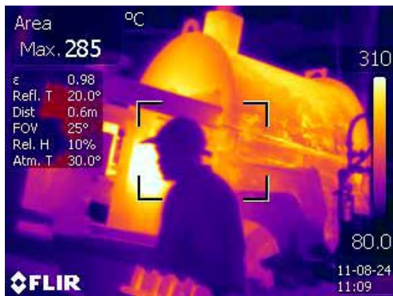
A thermal image taken at one of the participating foundries showing areas of heat loss on an aluminium casting furnace.
