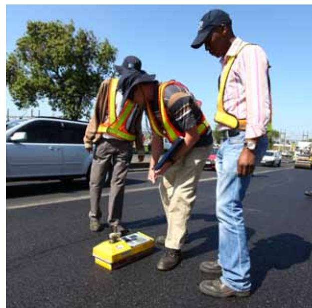
A density gauge is used to measure the density of the compacted high-modulus asphalt layer; optimal density ensures optimal performance.
