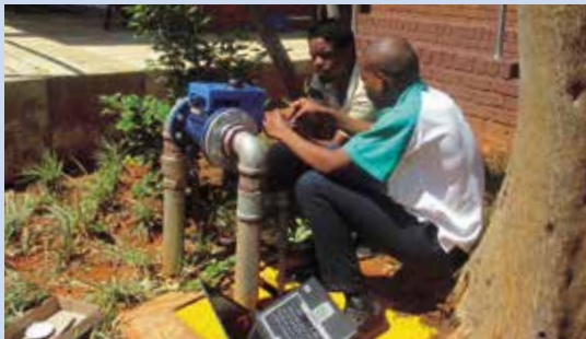
CSIR interns Mla Vilakazi and Matome Montja installing the SmartSense technology to monitor 33 water meters and three pressure sensors on the CSIR campus in Pretoria.
