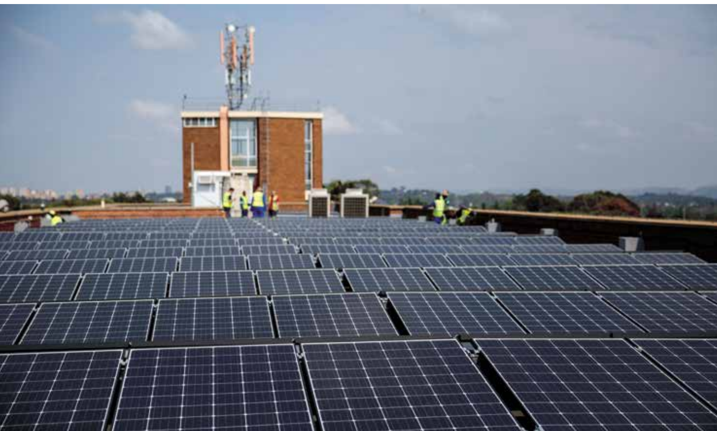
The CSIR completed the installation of a photovoltaic facility on the rooftop of one of the buildings on its Pretoria campus.
