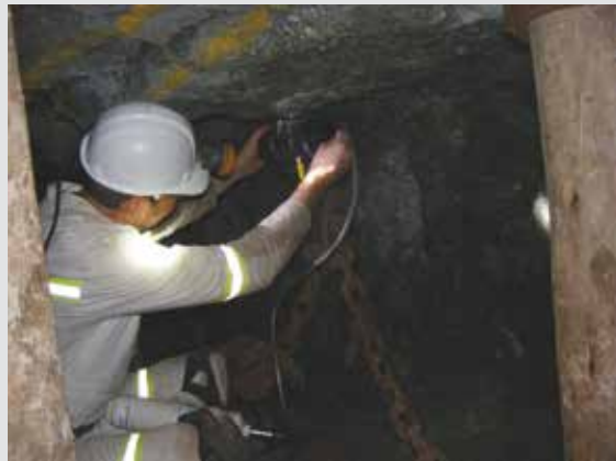
A CSIR engineer installs a wireless sensor in a platinum mine stope.
