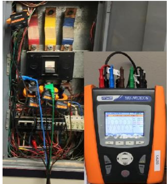
Fig. 2. HT Solar300N PQA connected at the main DB of the building
