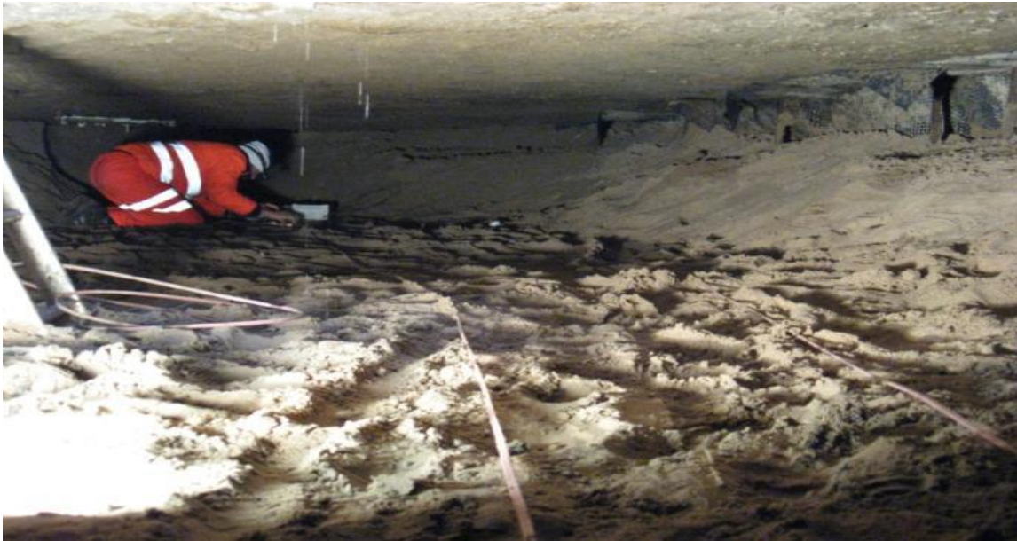
Figure 5: Soil erosion from underneath a Rotterdam quay wall
