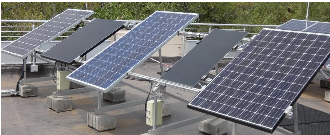
Figure 1: Different PV technology modules under test at Pretoria campus
