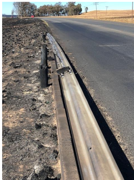
FIG. 3. DAMAGE TO GUARDRAIL AND BITUMINOUS SURFACING CAUSED BY WILDFIRE
