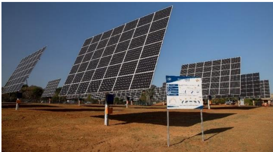
Dual-axis system 714 modules 202kWh capacity.
