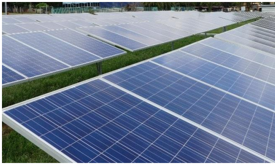
Single-axis system 1800 modules 558 kWh capacity.
