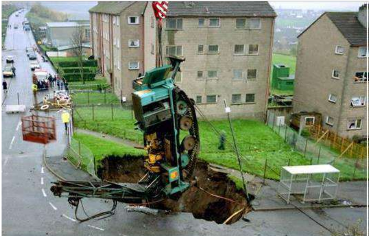
Figure 3: The underground of Glasgow city is full of old mine shafts. Not all are well mapped and accounted for. This drilling machine was mapping the quality of the subsurface when it occasionally found an abandoned mine shaft and fell in. Photo: British Geological Survey.
