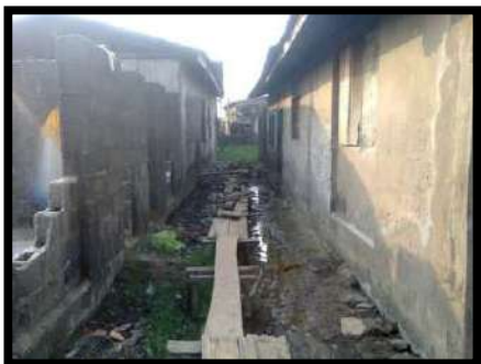
Photo 2: Clogged drainage between houses
