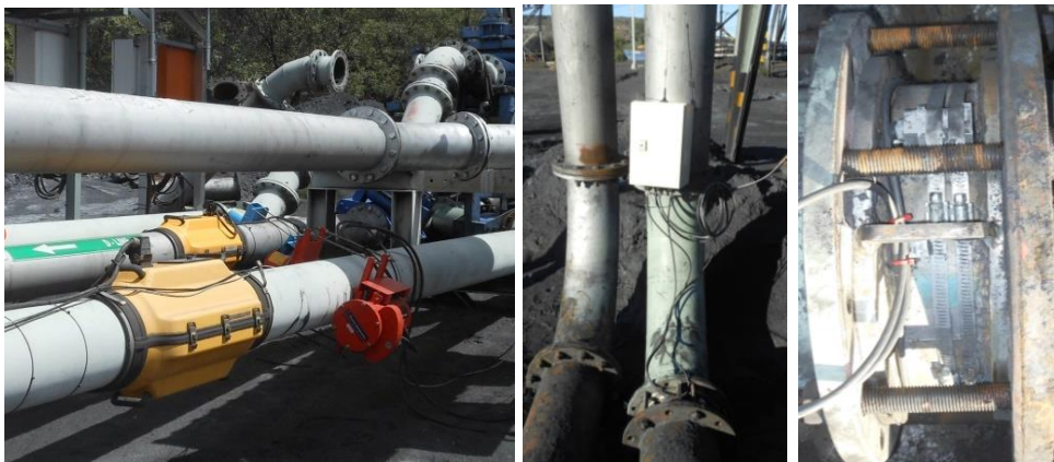
Figure 5 Flow meter, inclined density meter, control unit and installed short spool piece
