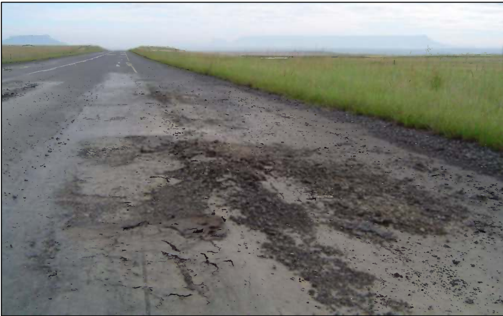
Figure 1: Heavy vehicle overloading contributes to accelerated pavement deterioration, which not only increases the cost of road maintenance (exponentially) but also increases vehicle operating costs.
